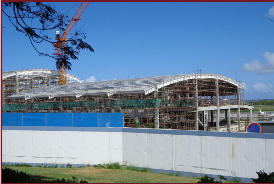
A view of the new terminal at V.C. Bird International Airport in Antigua, being built with assistance from the China Civil Engineering Construction Corporation. Photo: IPI.
